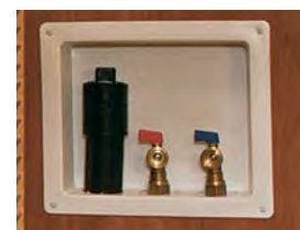
Residential washer/dryer hook-up in laundry closet.
